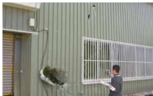
Photo. Collapse of wind power plant and damage to wall by a missile (at Miyakojima, T0314)
