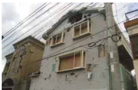
Figure 6 Damage to wall and roof
