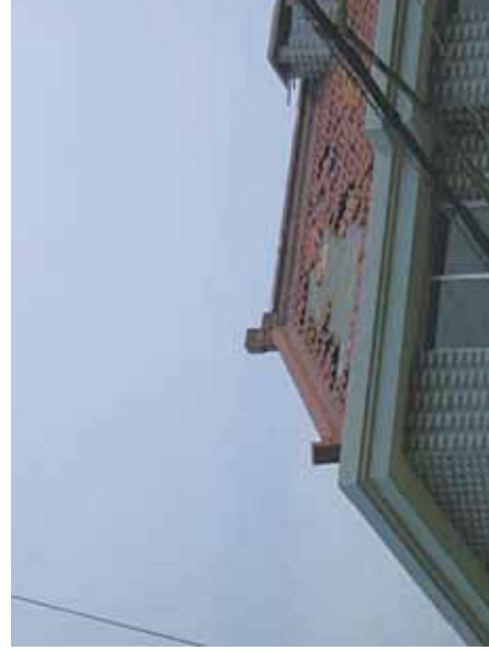
Photo 8. Damage to sloping roof
