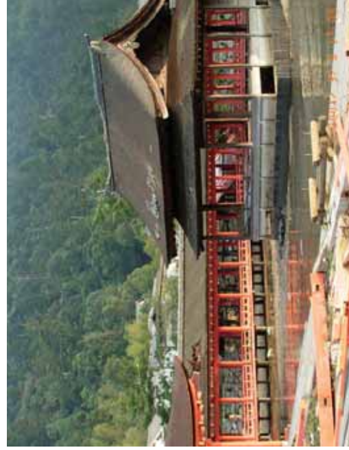
Photo 13. Separated roof tiles and damaged thatched roofs on leeward side
