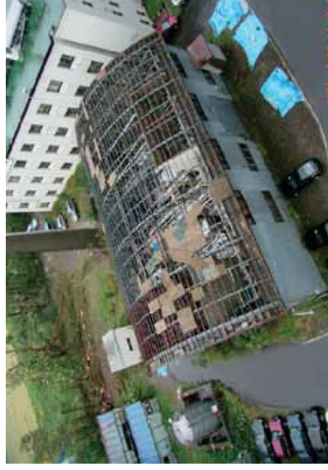
Photo 14. Damage to roof tiles (Hokkaido University)
