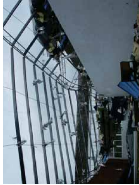
Photo 7. Broken steel roof
