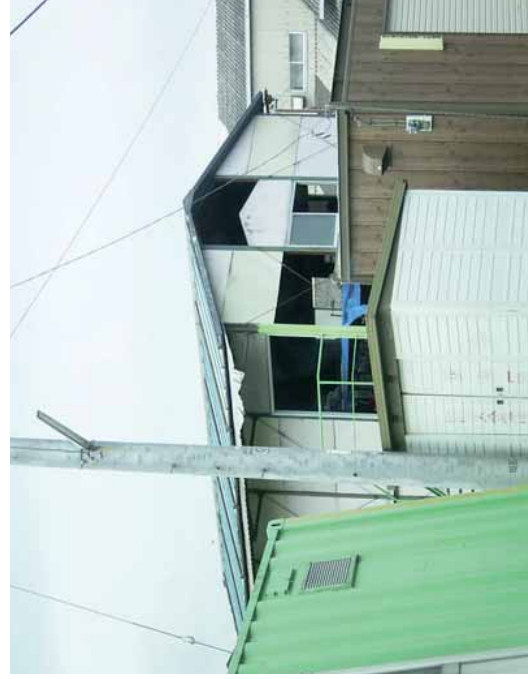
Photo 17. Broken wall of a factory building
