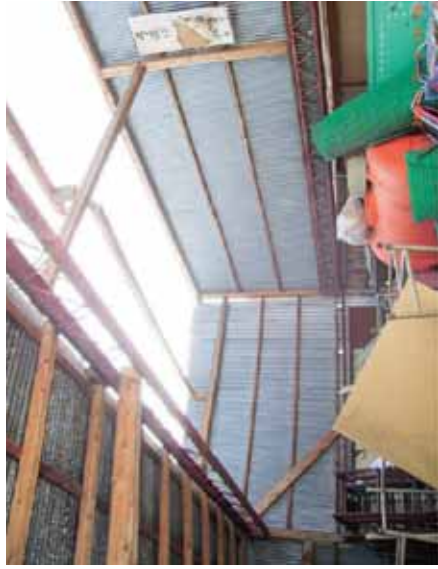
Photo 5. Roof blown off stock shed
