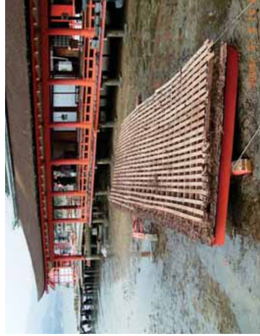
Photo 11. Damaged roof of corridor
