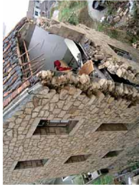
Photo 9. Collapse of stone wall of house
