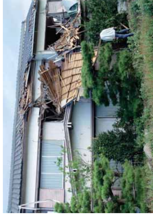
Photo 19. Cladding damage caused by flying debris
