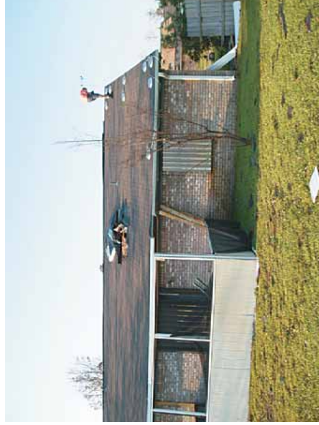
Figure 2. Photograph of Instrumented House with Roof of Porch and Chimney Damage
