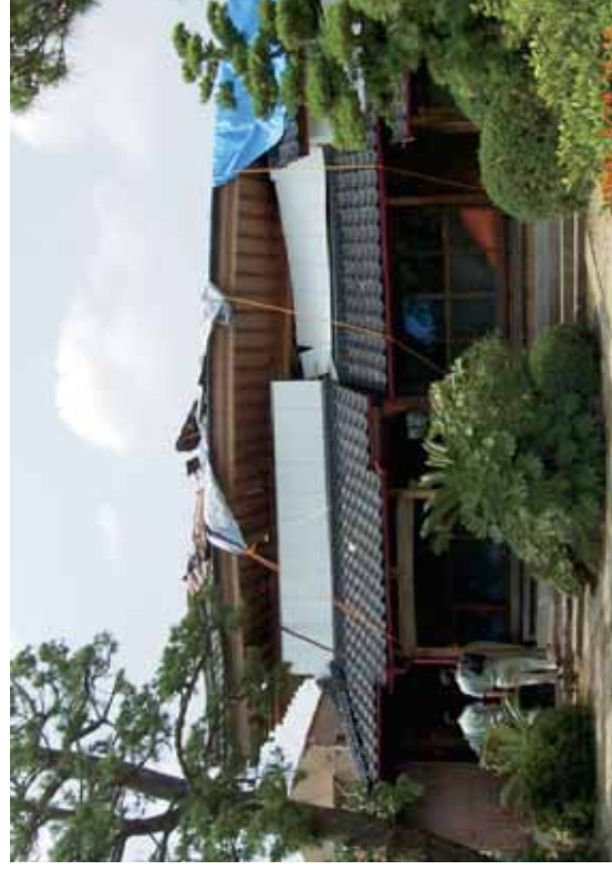
Photo 2. A damaged roof frame
