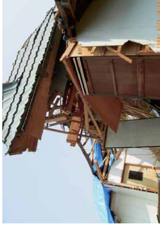
Photo 3. A collapsed wooden house
