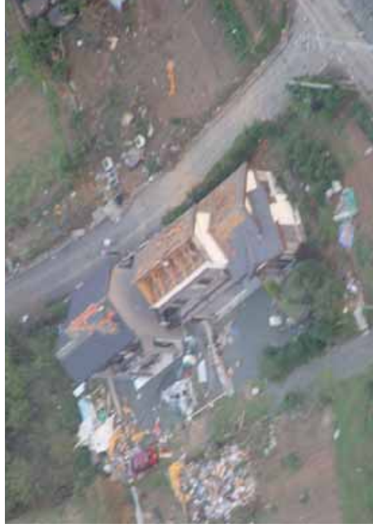
Photo 18. Roof damage to a residential house
