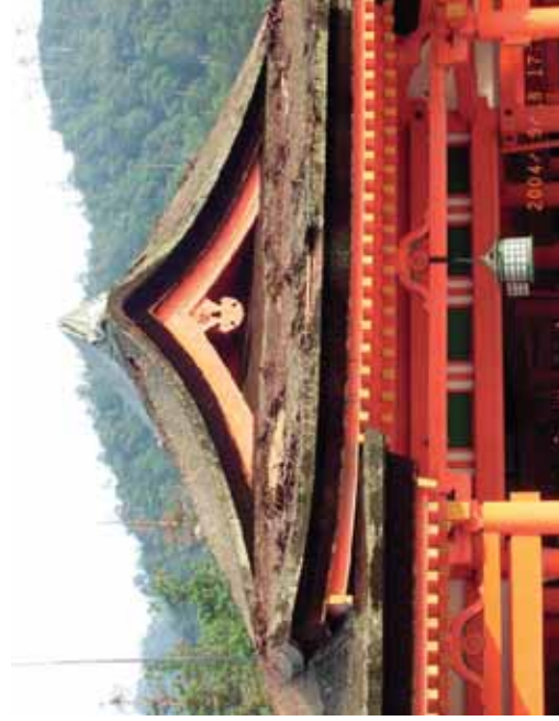
Photo 12. Damaged traditional thatched roof
