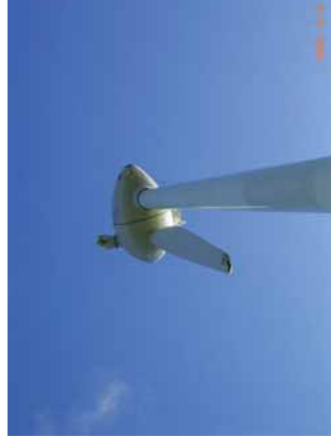
Photo 4. Damages to blades of a wind power plant
