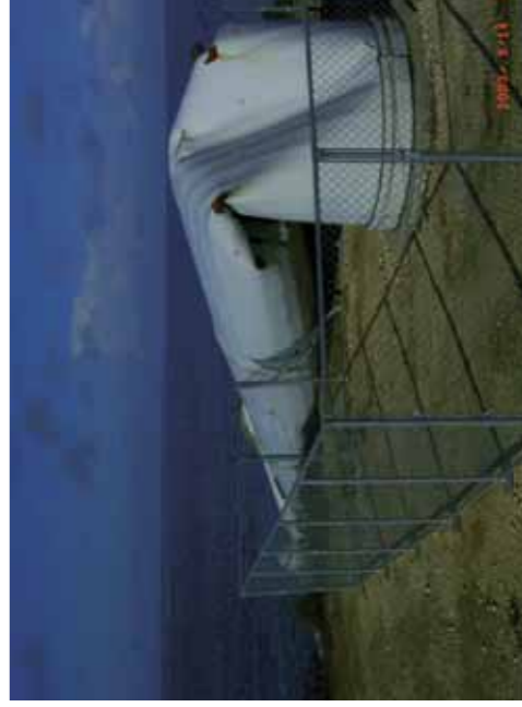
Photo 3. Collapse of wind power plant
