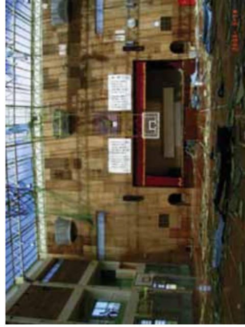
Photo 1. Damaged roof of a gymnasium
