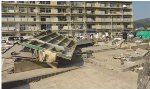
Fig. 12(b) Apartment damaged by debris.
