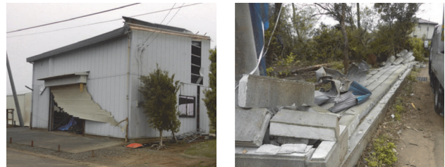
Fig. 5 Damaged storage structure and colapsed wall
