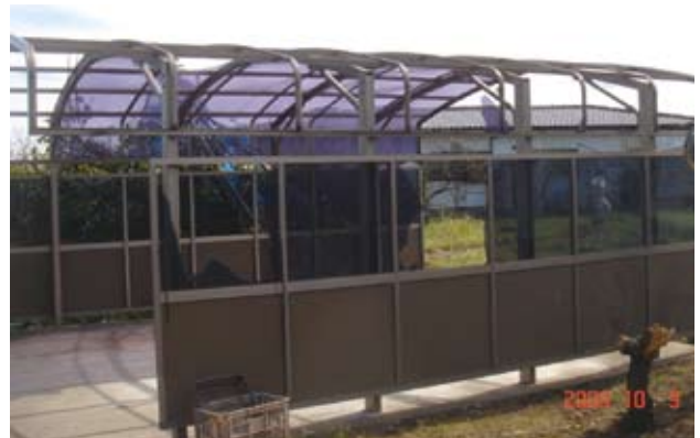
Fig. 15 Damaged roof of car garage
