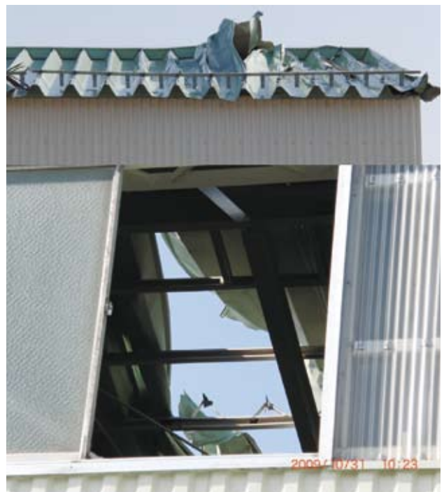
Fig. 27 Damaged roof steel sheet (point C)
