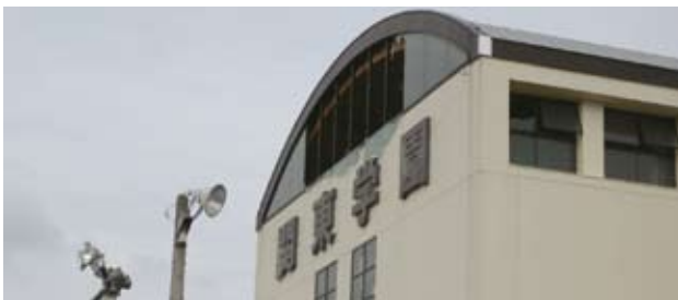
a. Damaged window of gymnastic hall (point C)
