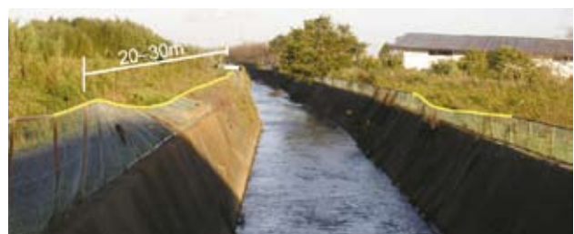
e. Inclined fences (damaged part described as yellow line)
