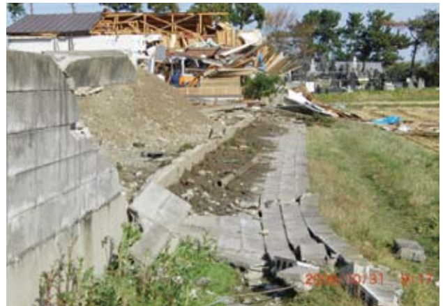
Fig. 25 Damaged Concrete Wall (point A)
