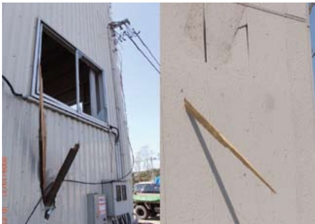
Fig. 28 Cladding damaged by debris (point C and B)
