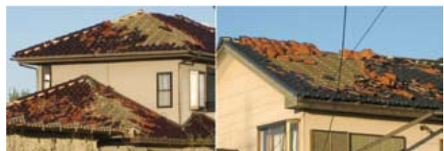
f. Damaged roof tiles
