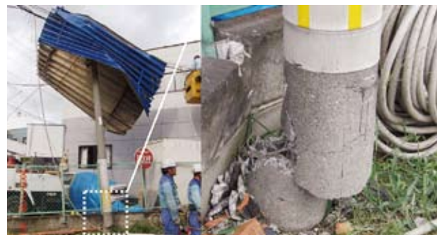
e. Damaged power pole due to debris (area A)
