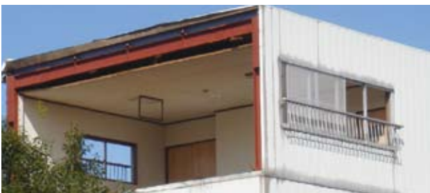
Fig. 17 Wall of steel structure blown away
