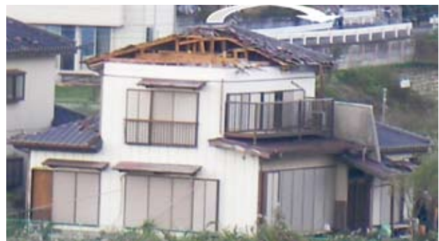
d. Window was broken and Roof structure blown off
