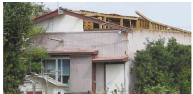
f. Damaged Roof truss (area B)
