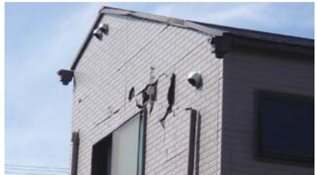
Fig. 14 Cladding damaged due to debris
