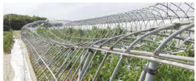
g. Damaged green house (area B) Fig. 20 Major damage due to tornado
