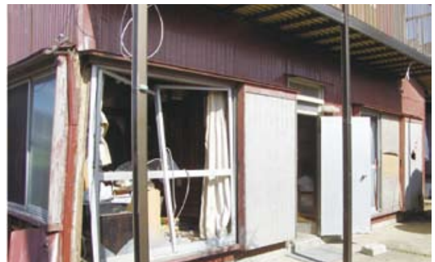
e. This dwelling was lifted up and down instantaneously by tornado (area A))
