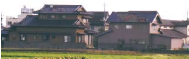
a. Damage to roof tiles
