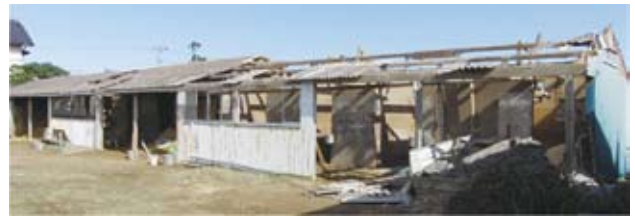
c. Damaged wooden cow house (area A)
