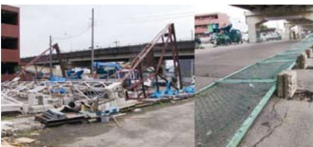
c. Fallen crane and fence (point A)
