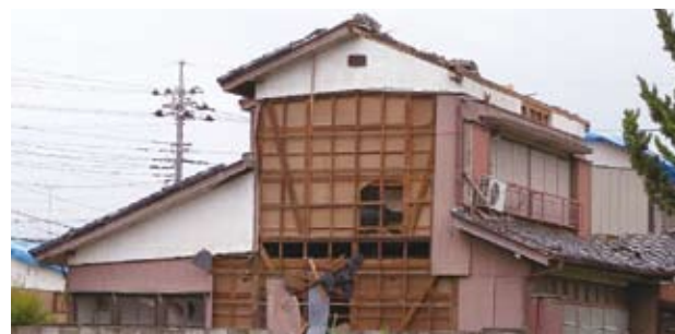
f. Damaged cladding (area A)
