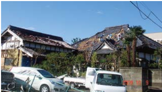
Fig. 11 Roof tiles of residential building blown away at touchdown point
