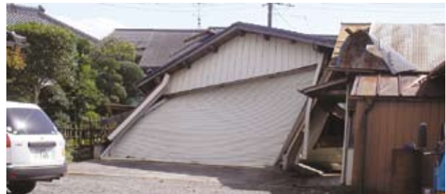
b. Collapsed garage
