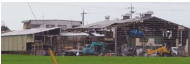
b. Wall of factory was flown away (point D)
