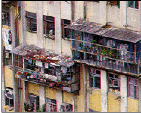
Figure 4: Building deterioration caused by Unauthorized Building Works (after Buildings Department, HKSAR)
