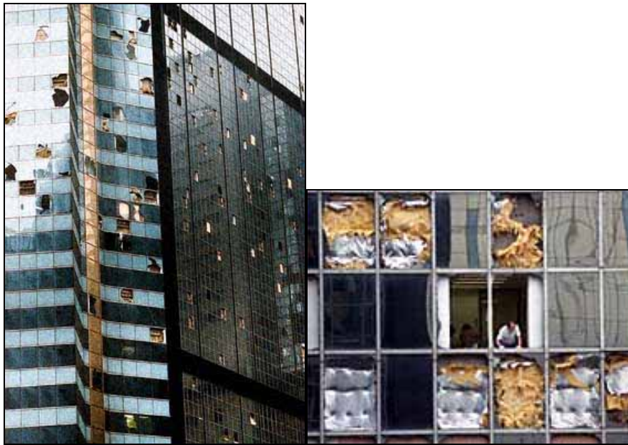
Figure 24: Cladding damage in the Wan Chai district of Hong Kong during Typhoon York (left), and a close-up of the damage (after van der Woning)
